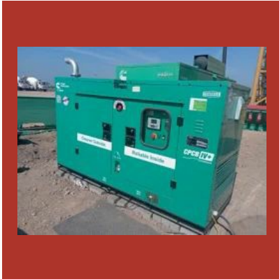
62.5 kVA Cummins Silent Diesel Generator
