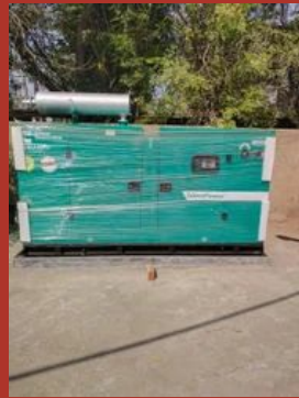
Cummins 15 kVA Single Phase Diesel Generator
