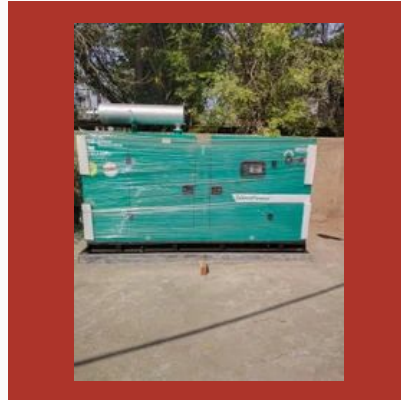
Cummins 10 kVA Three Phase Diesel Generator in UAE
