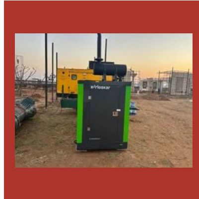
7.5 kVA KOEL by Kirloskar Air Cooled Diesel Generator
