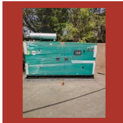
35 kVA Cummins Silent Diesel Generator
