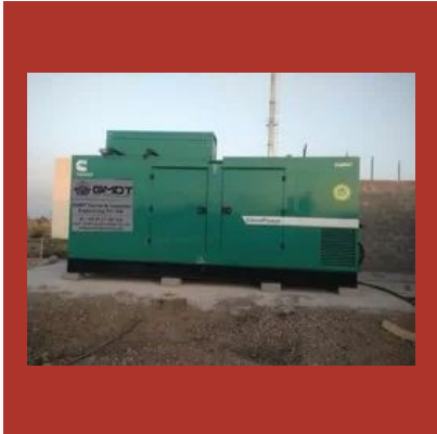
Three Phase Generator
