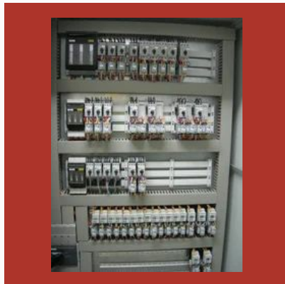
Electrical MCC Panel
