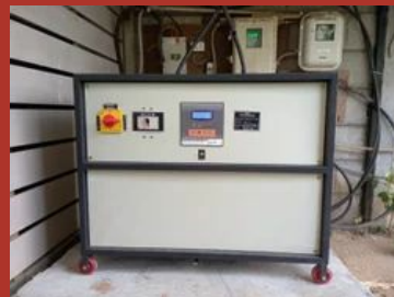
45 KVA 3 Phase Servo Voltage Stabilizer
