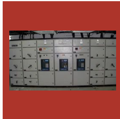
LT Distribution Panel
