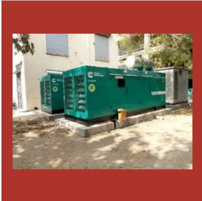
910 Kva Sudhir Diesel Generator
