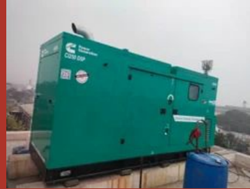
High efficiency diesel generator in Iran
