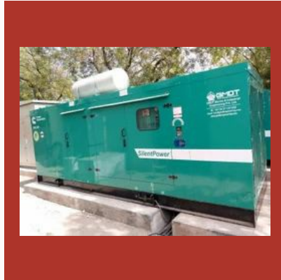
Sudhir 125 KVA Diesel Generator
