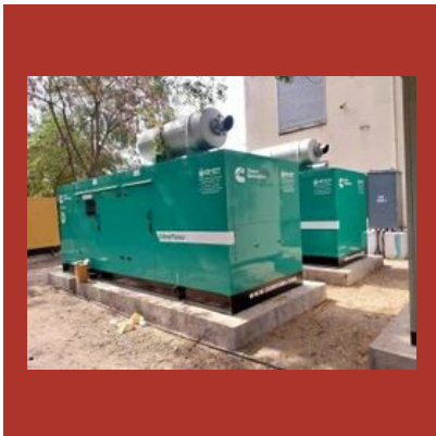
20 kVA Cummins Silent Diesel Generator
