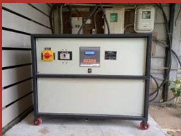
40 KVA 3 Phase Servo Voltage Stabilizer
