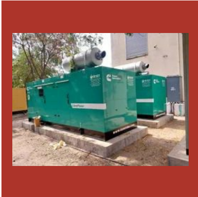
50 KVA Mahindra Powerol Generator
