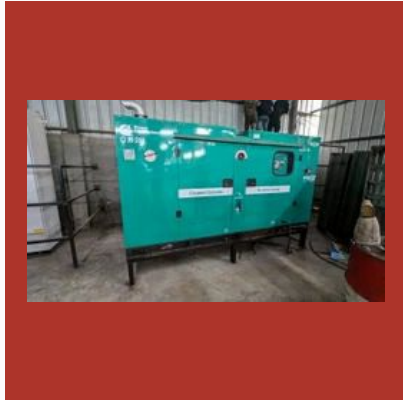
Commercial diesel generator in Iran
