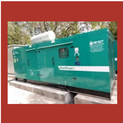
Sudhir 7.5 KVA Diesel Generator
