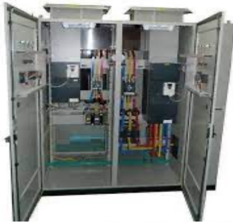
VFD panel (Variable Frequency Drive)
