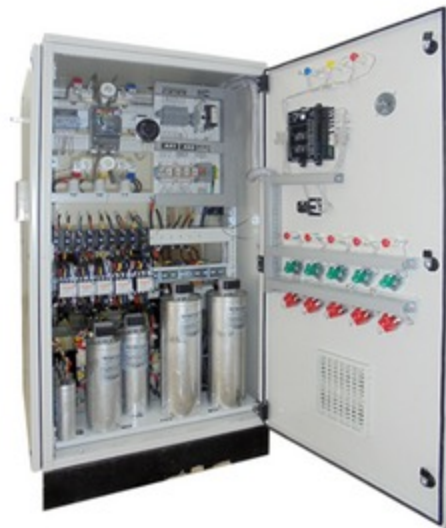
APFC (Automatic Power Factor Correction panel)
