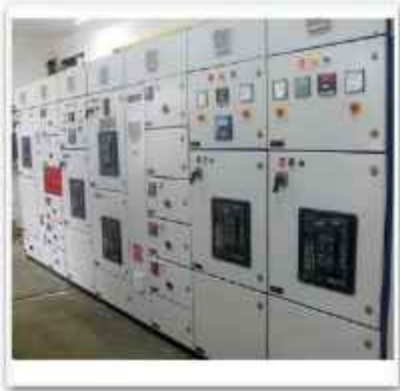
LV Power Control Center
