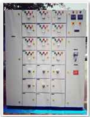
Motor Control Center
